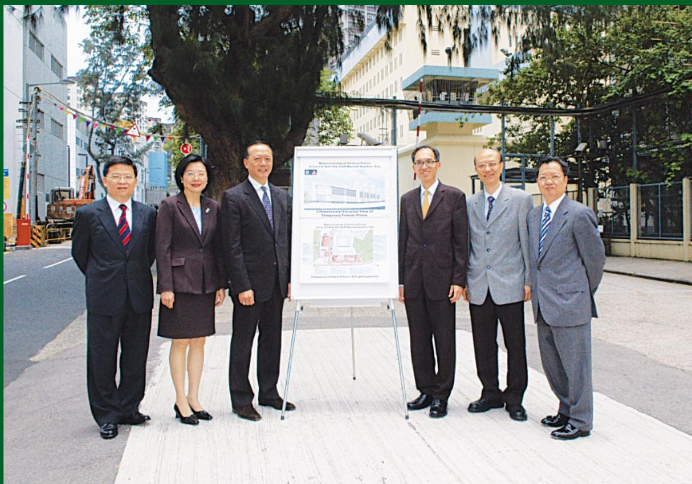
政務秘書黃永康 (右三) 及團隊巡視荔枝角收押所工程。 Mr Stanley Wong (third from right), Civil Secretary, and supporting team inspecting the construction project at Lai Chi Kok Reception Centre.
