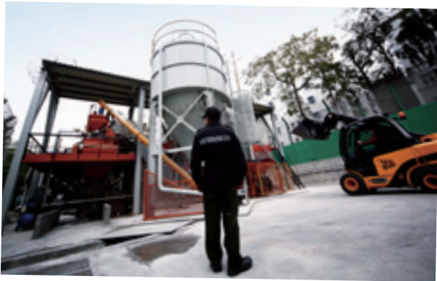
大榄惩教所更换新的混凝土物料调配设施。 An aged concrete batching plant at Tai Lam Correctional Institution is replaced to improve production efficiency.
